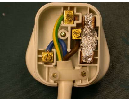
Fuse not being used.
