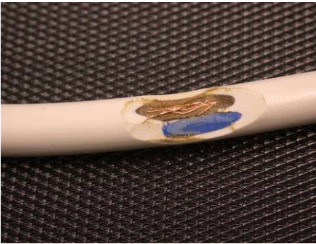
Damage to power cable sheath.
