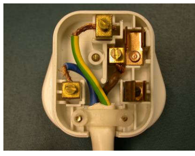
Bare wires visible.
