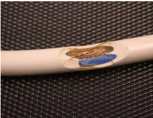
Damage to power cable sheath.
