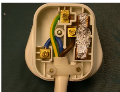
Fuse not being used.
