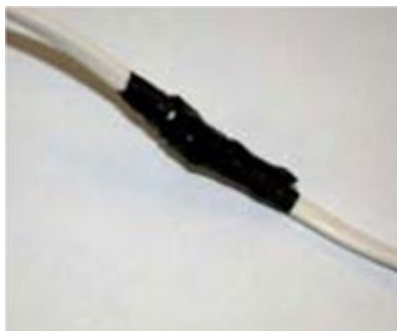
1b Taped joint of cable
